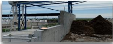
AMMP Project: Glenn County
