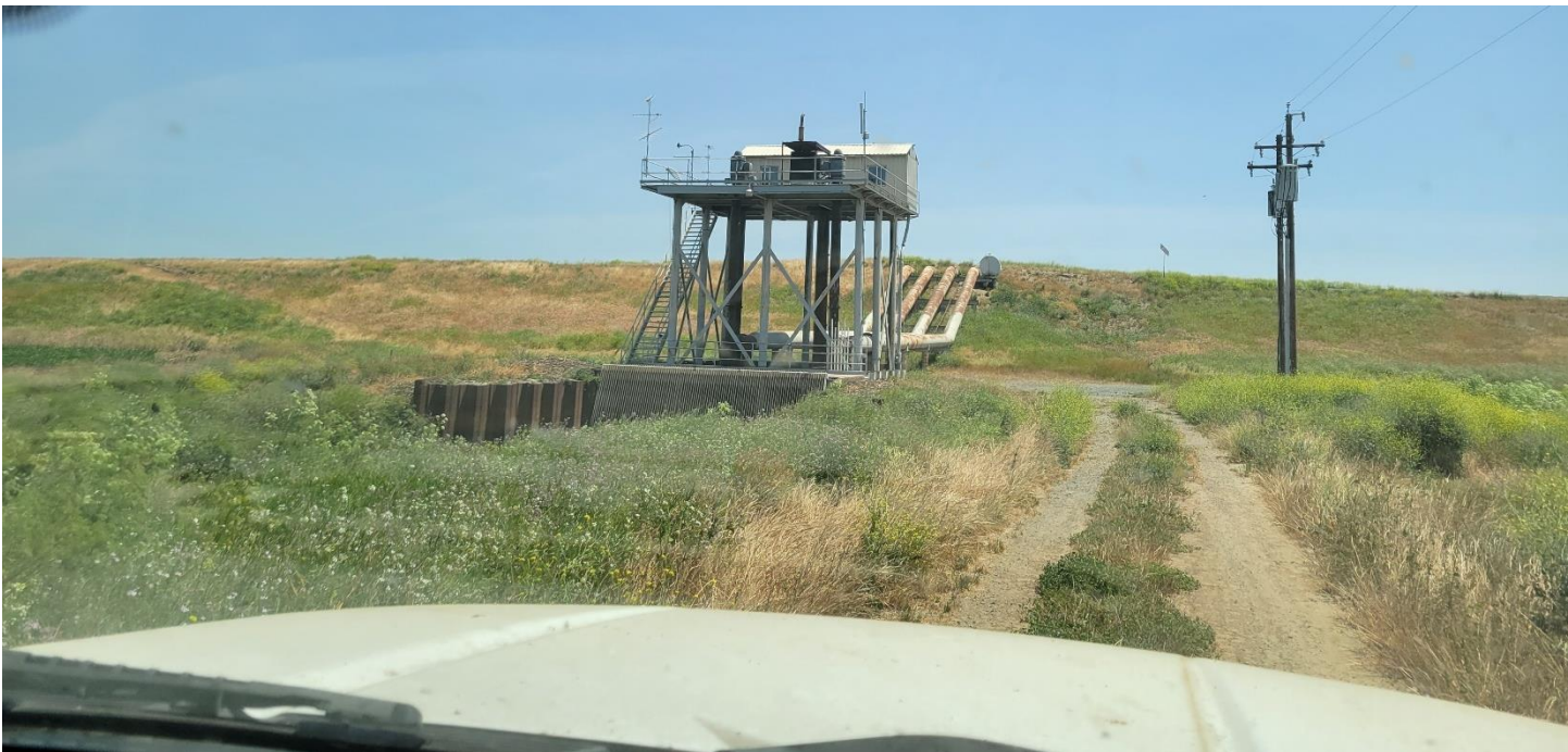
Figure 3. South Pump at Staten Island
