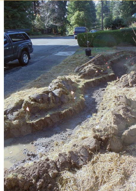
Figure 5. Gravel has been added to the bottom of the streambed during this construction in this home yard. Source: High Tide Permaculture
