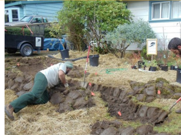
Figure 3. Removing a lawn and creating a channel for water flow. Source: High Tide Permaculture
