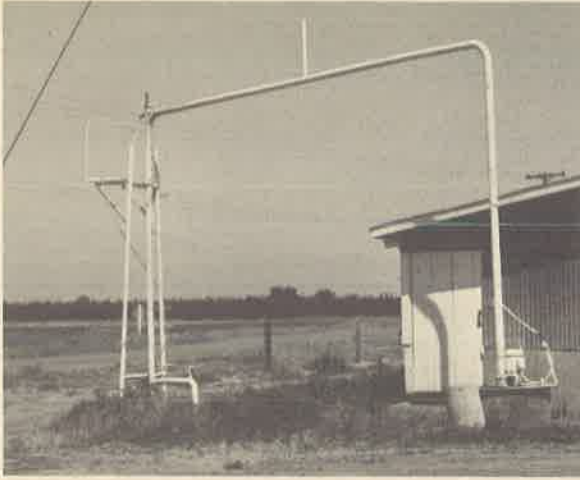
Wastes are collected in a sump and then pumped into irrigation pipeline for distribution.
