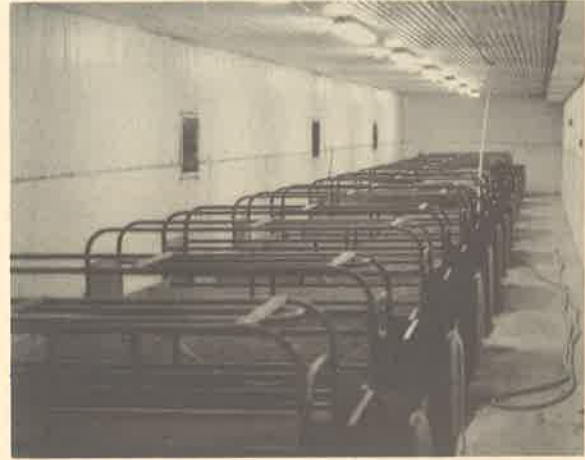
Interior view of a 16-crate farrowing barn. This is one of four individual barns. Farrowing is carried out in three while the fourth is depopulated and disinfected. These units have radiant heat in floor.
