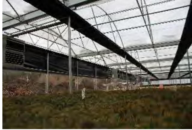
Figure 6.3 A double-layer polyethylene gutter-connected greenhouse designed to grow tree seedling in California. Note the roll-up walls and the black-cloth system for dormancy induction using shortened photoperiod. There are also lights to extend the photo period.
