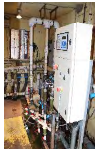
Figure 6.4 Irrigation pumps and fertilizer injector.
