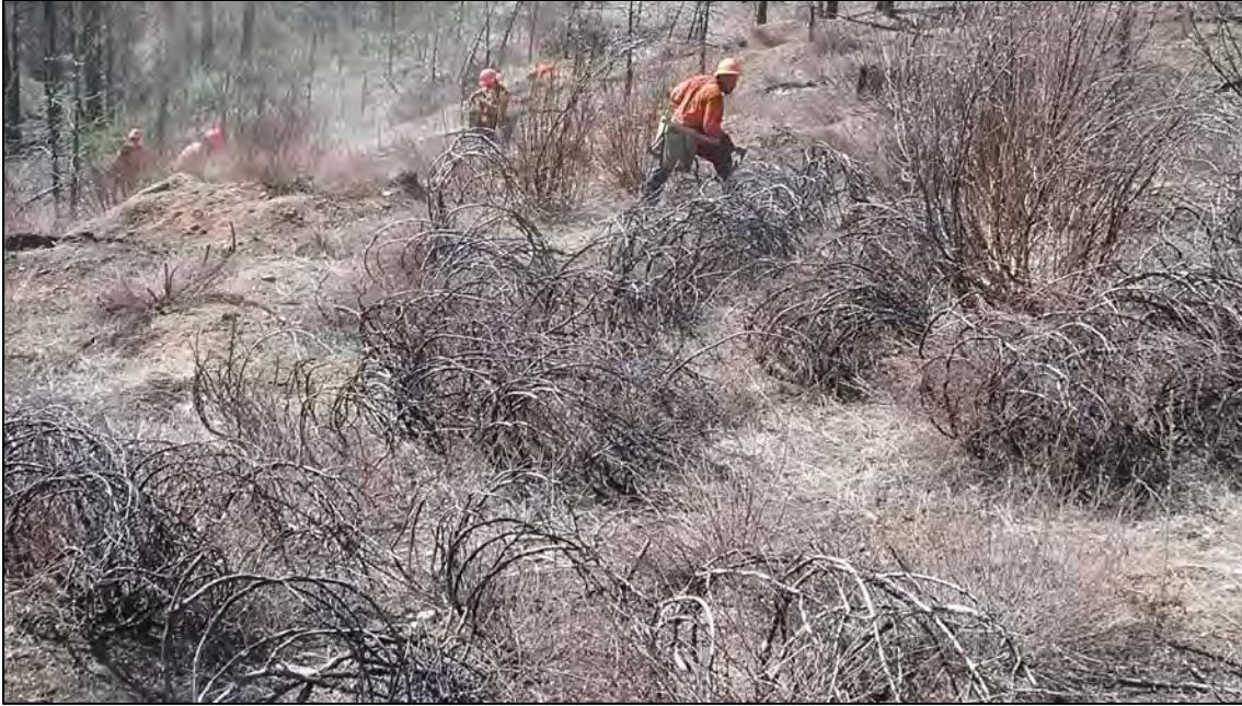
Figure 9.6 Dead brush skeletons also provide suitable shade for Douglas-fir (DF) and white fir (WF) seedlings during the critical first summer growing season after planting. Crews are instructed to plant ponderosa pine in openings and DF and WF in partial shade of dead brush where feasible to reduce direct solar radiant heat on the sensitive basal stems of these species. By the time winter snow crushes down the brush skeletons, the DF and WF seedlings will be sufficiently developed to withstand direct sunlight.
