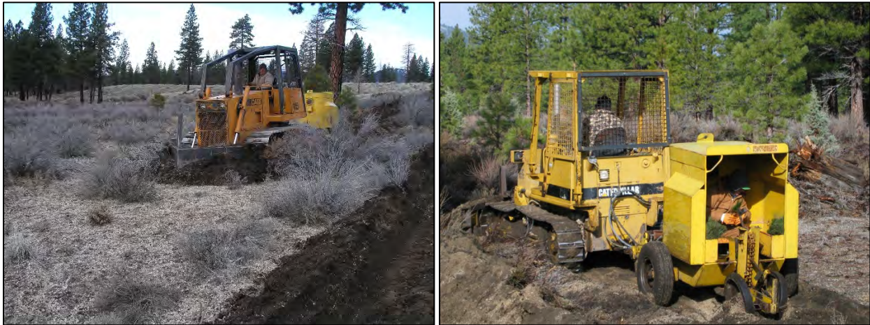
Figure 9.12 A “V Blade” attached to the front of a crawler tractor scalps away grass and brush making a level surface of moist mineral soil (left) in preparation for planting 2-0 bareroot ponderosa pine seedlings by the planting machine attached behind the crawler tractor.
