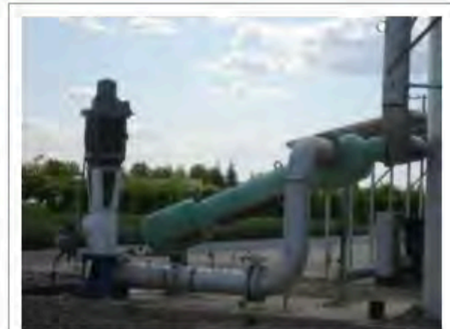
Groundwater well with sand separator Photo: L. Schwankl
