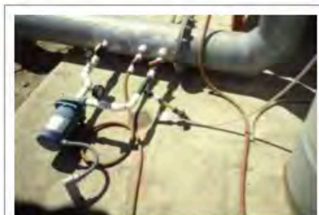
Venturi injector with small pump. Photo: L. Schwankl
