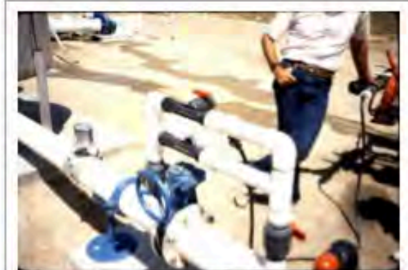
Double-venturi injection system Photo: L. Schwankl
