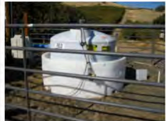
Storage tank for chemicals injected through the microirrigation system Photo: L. Schwankl
