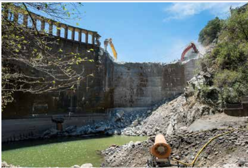
Demolition of the 106-foot-high San Clemente Dam on the Carmel River. Photo: California American Water
