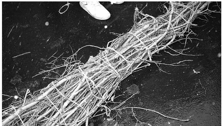
Below, bundles of dormant willows tied into a willow wattle ready for installation across a steep slope.
