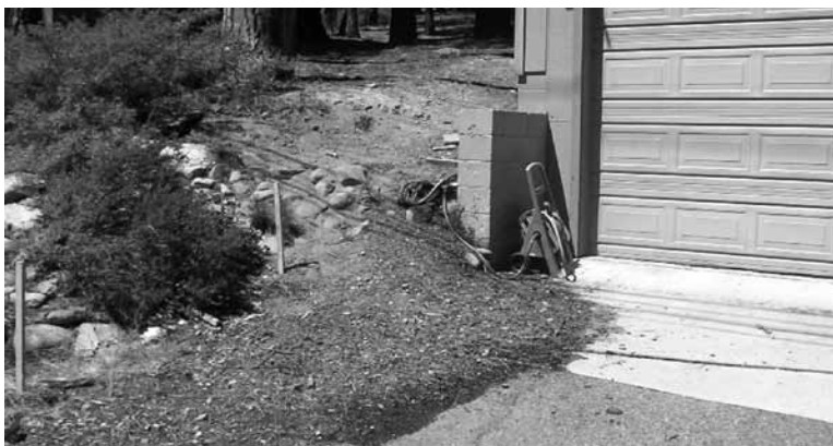
Poor erosion control and an inefficient retaining border allows sediment to spill onto driveway, which will prematurely clog the infiltration system.
