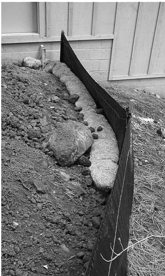
The silt fence and fiber roll log will remove sediment from runoff if a rainstorm occurs.
