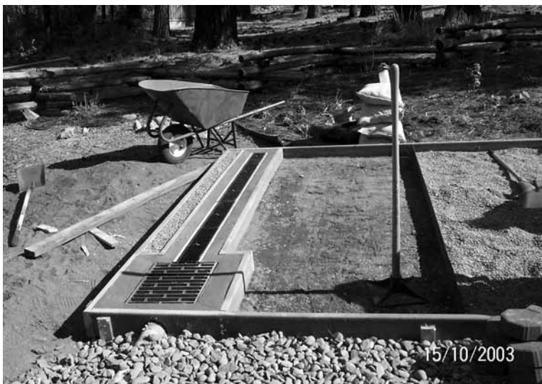
Pre-treatment sediment trap with large grate is easily cleaned.
