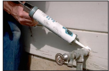
Figure 5. Caulking ant entryways is a key element of an ant IPM program.
