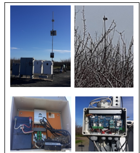
Figure 7. Parts of a telemetry system. Cell tower and gateway next to pump controls (top left), gateway connection to internet (bottom left), orchard cell tower connected to sensors in the field (top right); and node connection to field sensors (bottom right).
