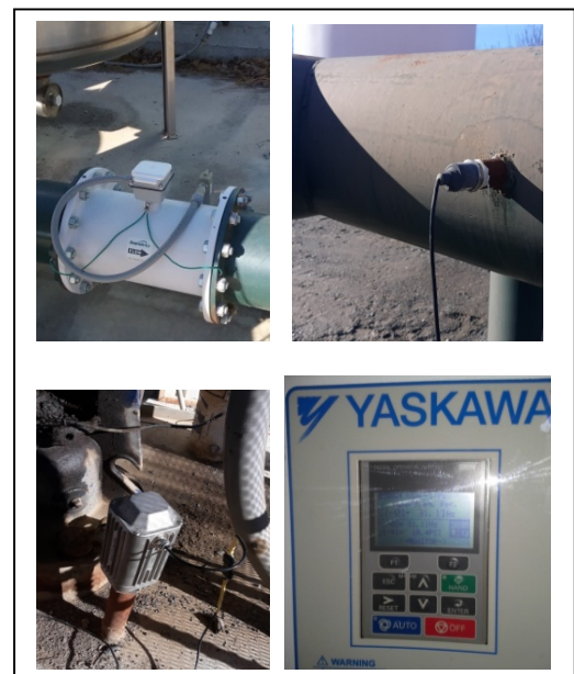
Figure 3. Magnetic flow meter (upper left), pressure transducer (upper right), acoustic groundwater level sensor (lower left), and VFD digital control panel (lower right).
