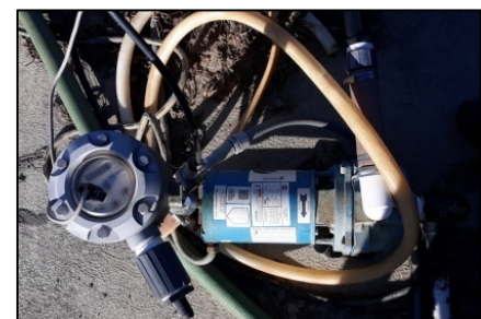
Figure 5. Pressure transducer on irrigation line (top) and flow meter on injection pump (bottom).
