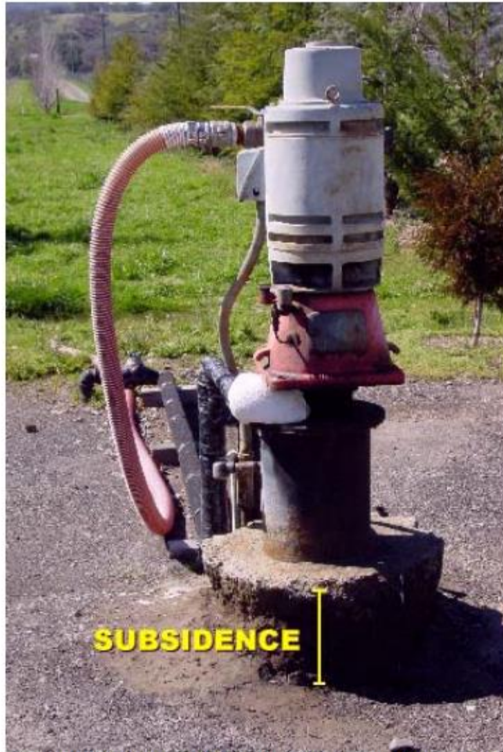
A groundwater well along Scotts Valley Road, showing subsidence around the well collar.
