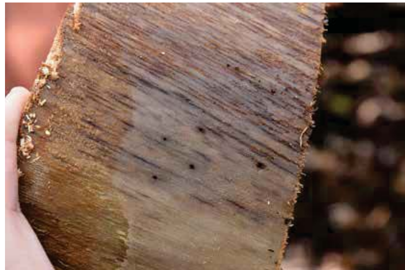
Photo 5. Small, dark holes in the sapwood further indicate wood boring beetles are present. Photo by Sonia Rios
