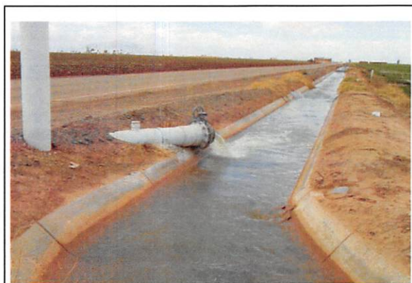
Figure 3. Circulation collected water around field through tailwater recovery system
