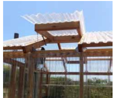
Vents in a greenhouse roof should allow for opening of at least 20% of the roof area
