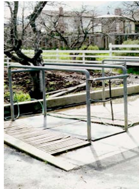
A curb directs horse wash water away from the creek. Keep horse wash water out of creeks, seasonal drainages, and storm drains. Horse wash areas should be kept clean of manure and grooming products.
