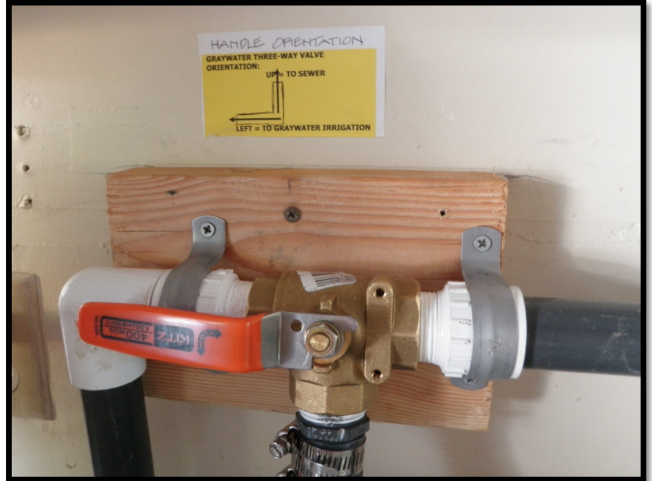
3-way valve for laundry waste water
