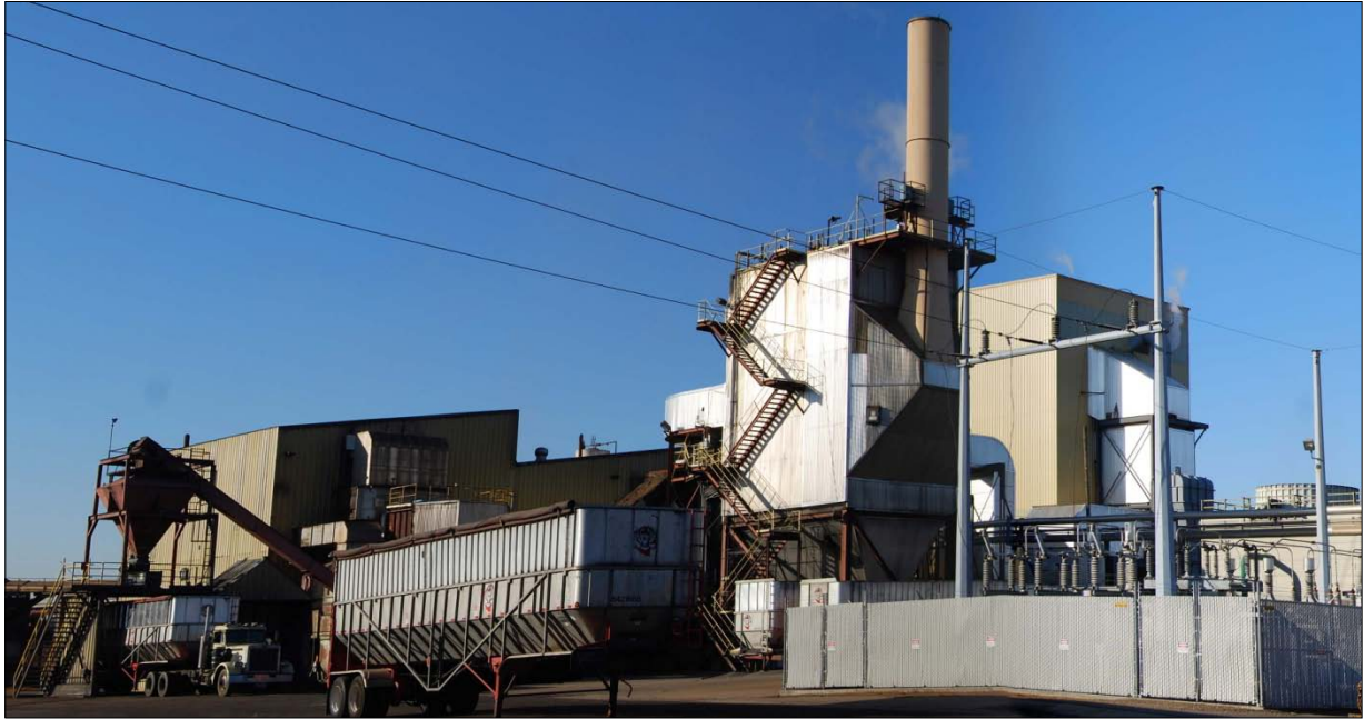
SPI Lincoln Biomass energy recovery cogeneration recovery steam boiler facility.
