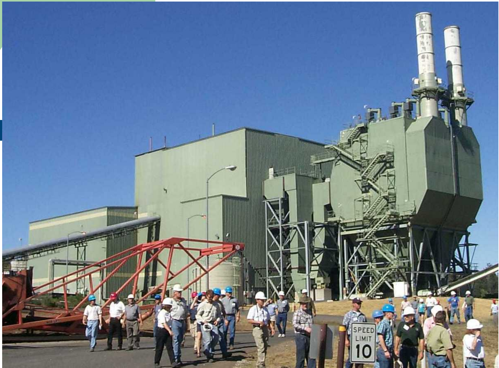
Burney Forest Power 31 MW CHP at Burney, CA
