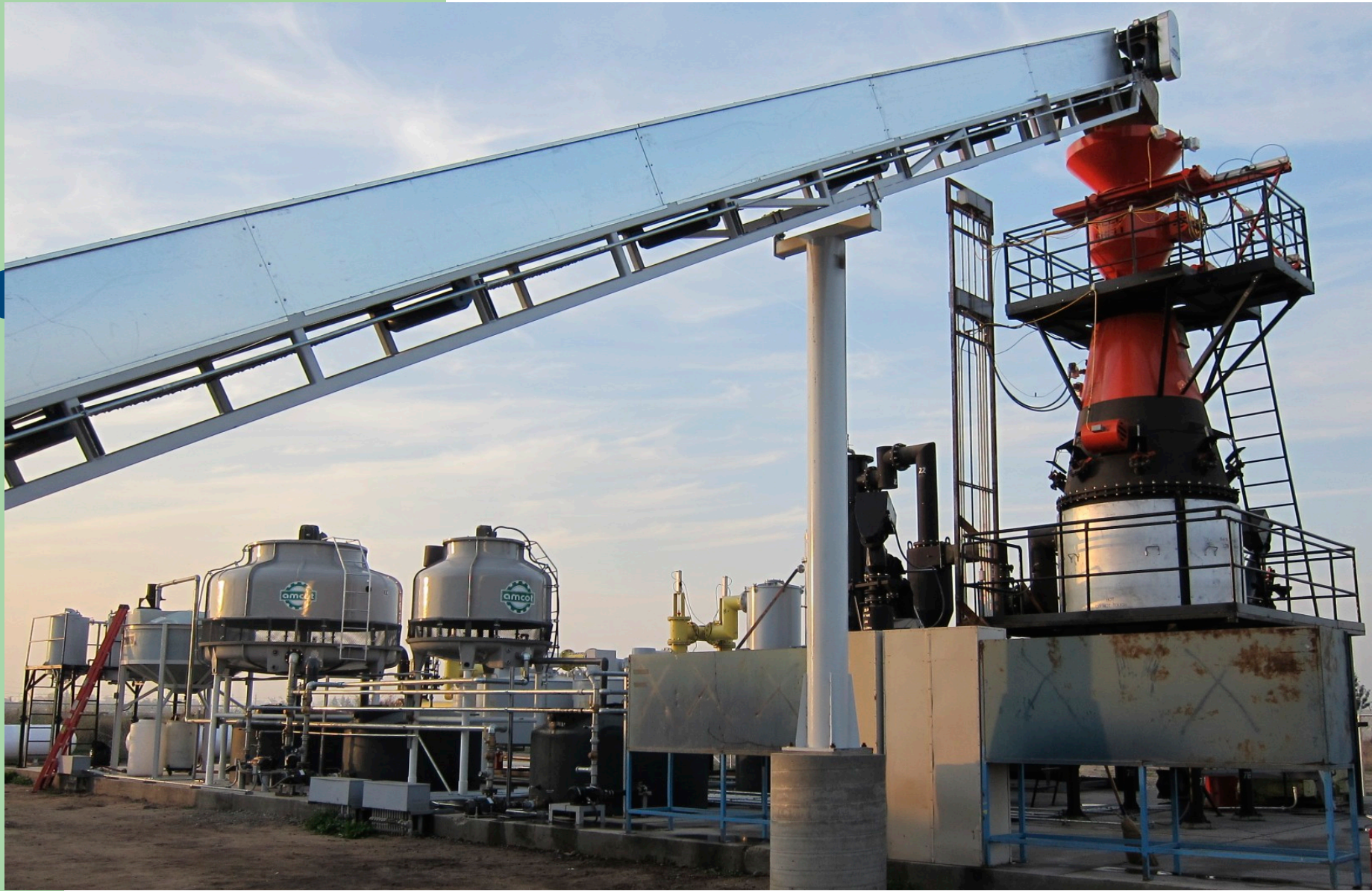
Phoenix Energy 500 kWh Gasification Unit at Merced, CA
