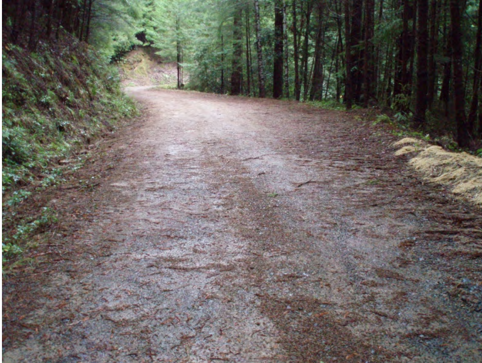
Figure 1 —Site 8, December HY07, showing rocked road surface following summer grading.
