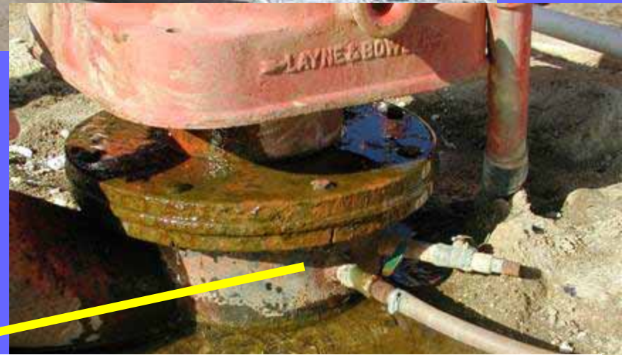
Injection nipple on well casing dribbling chemicals directly into groundwater.
