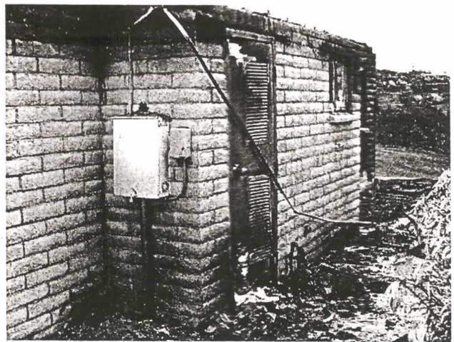
Figure 4. ~ Vents located on an exterior door possibly contributed to loss of this structure by allowing burning embers into the room containing mechanical equipment.
