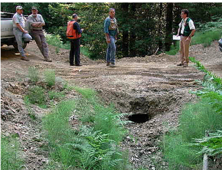
Figure 16. Culvert plugged with sediment at inlet. Photo: Angela Wilson, Central Valley Regional Water Quality Control Board.
