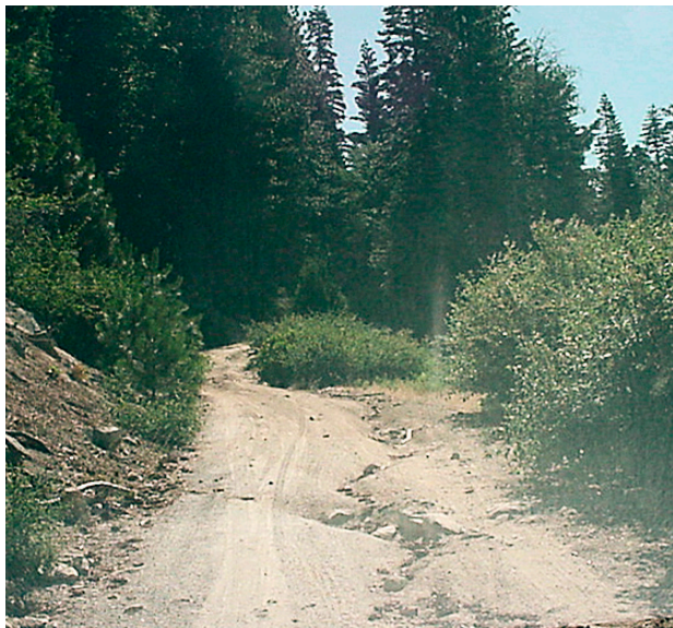
Figure 37. Pinchard Creek road with rilling along the road surface before the project, 2002. Photo: Joe Hoffman, Plumas National Forest.
