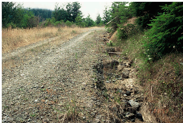
Figure 20. Eroding inboard ditch on an in-sloped road. This is a symptom of inadequate cross drains for conveying ditch flow across the road. Photo: Richard Harris.
