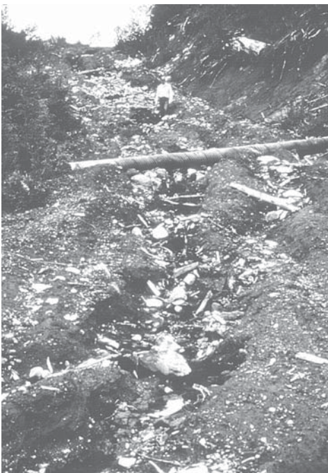
Figure 6-10. Catastrophic ditch and roadway erosion.
