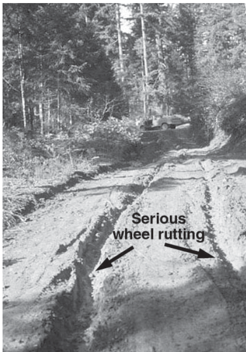
Figure 6-2. Excessive wheel rut damage to the road surface.
