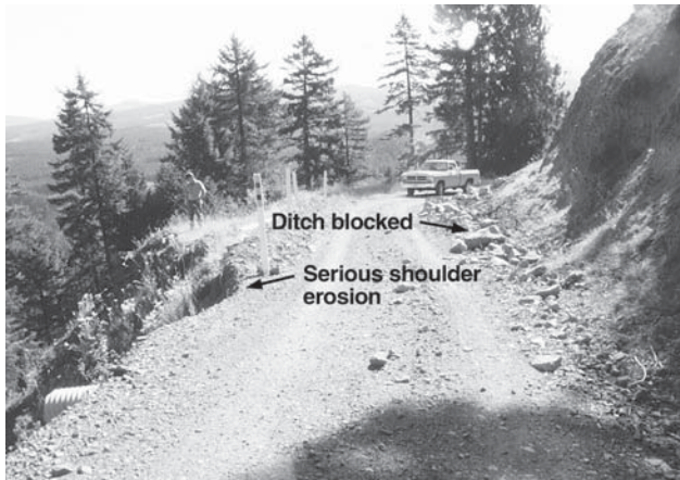
Figure 6-1. Roadway failure due to lack of proper maintenance.
