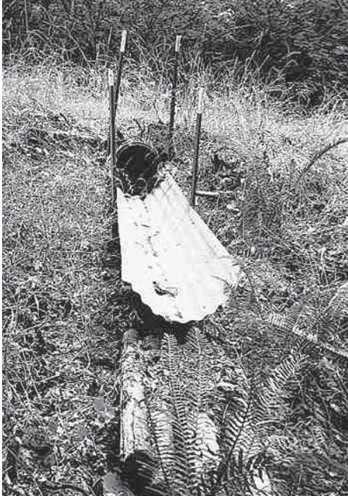
Figure 2-10. Downspout with corrugated metal roof sheeting, with slash logs for energy dissipation.
