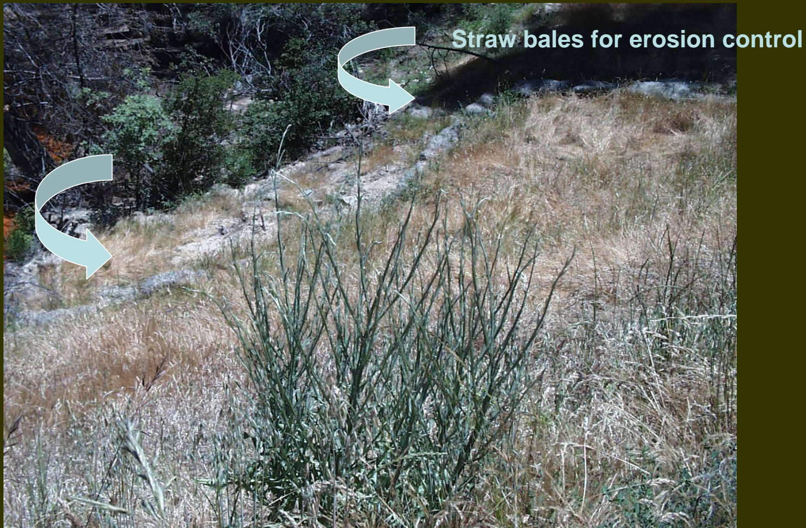
Madera County, Federal Highway Administration Chepo Saddle road reconstruction, Sierra National Forest June 2000 - 1 year after project completion
