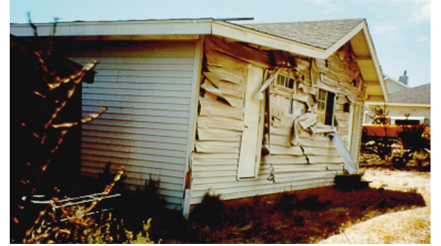
RADIANT HEAT melted this house's vinyl siding and window frames.
