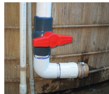
Firefighters' delight: a 10,000-gallon water tank with a valve and 2-1/2" National Hose male fitting, located where a fire engine can easily connect to it, full of water and ready to protect your home and property!
